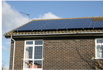
Figure 3. Solar photovoltaics: data from a 25\text{-m}^2 array in Cambridgeshire in 2006. The peak power delivered by this array is about 4\text{ kW} . The average, year-round, is 12\text{ kWh} per day. That's 20\text{ W} per square metre of panel.
