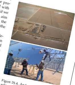
Figure 25.4. Andasol – a "100 MW" solar power station under construction in Spain. Excess thermal energy produced during the day will be stored in liquid salt tanks for up to seven hours, allowing a continuous and stable supply of electric power to the grid. The power station is predicted to produce 350 GWh per year (40 MW). The parabolic troughs occupy 400 hectares, so the power per unit land area will be 10 W/m 2 . Upper photo: ABB. Lower photo: IEA SolarPACES.
