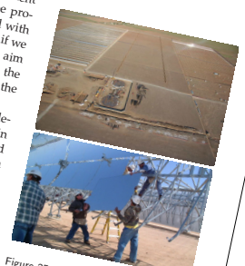
Figure 25.4. Andasol – a "100 MW" solar power station under construction in Spain. Excess thermal energy produced during the day will be stored in liquid salt tanks for up to seven hours, allowing a continuous and stable supply of electric power to the grid. The power station is predicted to produce 350 GWh per year (40 MW). The parabolic troughs occupy 400 hectares, so the power per unit land area will be 10 W/m 2 . Lower photo: IEA SolarPACES.
