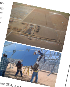
Figure 25.4. Andasol – a "100 MW" solar power station under construction in Spain. Excess thermal energy produced during the day will be stored in liquid salt tanks for up to seven hours, allowing a continuous and stable supply of electric power to the grid. The power station is predicted to produce 350 GWh per year (40 MW). The parabolic troughs occupy 400 hectares, so the power per unit land area will be 10 W/m 2 . Lower photo: ABB. Lower photo: IEA SolarPACES.
