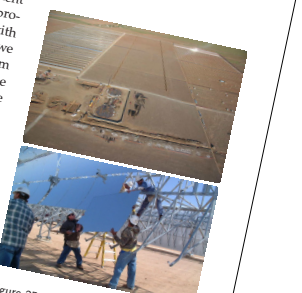
Figure 25.4. Andasol – a "100 MW" solar power station under construction in Spain. Excess thermal energy produced during the day will be stored in liquid salt tanks for up to seven hours, allowing a continuous and stable supply of electric power to the grid. The power station is predicted to produce 350 GWh per year (40 MW). The parabolic troughs occupy 400 hectares, so the power per unit land area will be 10 W/m 2 . Solar photo: ABB. Lower photo: IEA SolarPACES.
