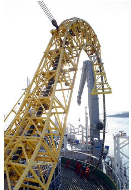
Figure 10. Laying a high-voltage DC link between Finland and Estonia. A pair of these cables transmit a power of 350 MW. Photo: ABB.
