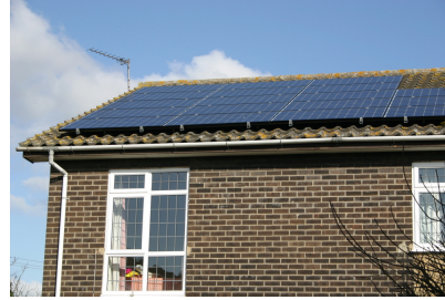
Figure 9. Solar photovoltaics: data from a 25-m 2 array in Cambridgeshire in 2006. The peak power delivered by this array is about 4 kW. The average, year-round, is 12 kWh per day. That's 20 W per square metre of panel.
