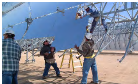
Figure 8. Andasol – a "100 MW" solar power station under construction in Spain. Excess thermal energy produced during the day will be stored in liquid salt tanks for up to seven hours, allowing a continuous and stable supply of electric power to the grid. The power per unit land area will be 10 \text{ W/m}^2 . Photo: IEA SolarPACES.
